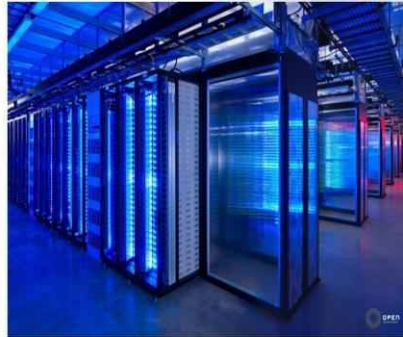
Facebook's datacenter facility in Prineville, Oregon runs on Open Compute Project hardware. Photo credit: Alan Brandt [ref] Open Compute Project http://www.opencompute.org/
