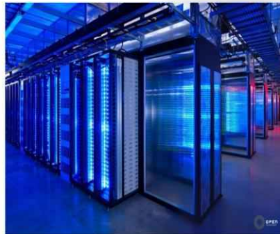
Facebook's datacenter facility in Prineville, Oregon runs on Open Compute Project hardware. Photo credit: Alan Brandt [ref] Open Compute Project http://www.opencompute.org/
